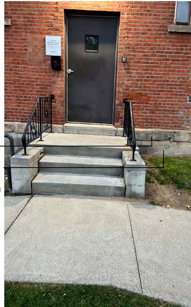
EXISTING STAIR: TO BE REMOVED
